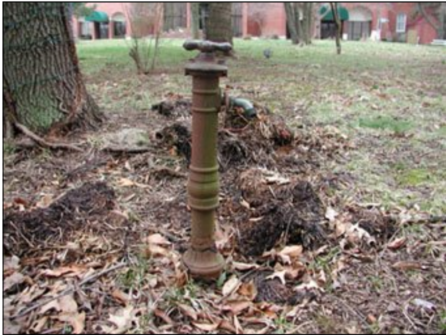
Early 1900's Yard Hydrant (Photo by Author)
