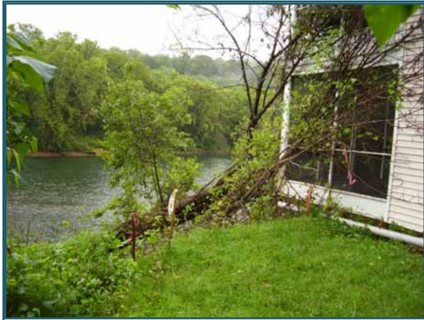
Picture 1. Bank erosion threatening an Ozark condominium building (2008 photograph by Olsson)
